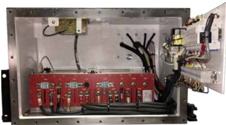
Q750 system mounted in XP box with swinging panel open
