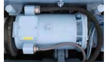
Mining locomotive motor installed
