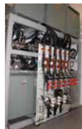
Stationary custom panel work
